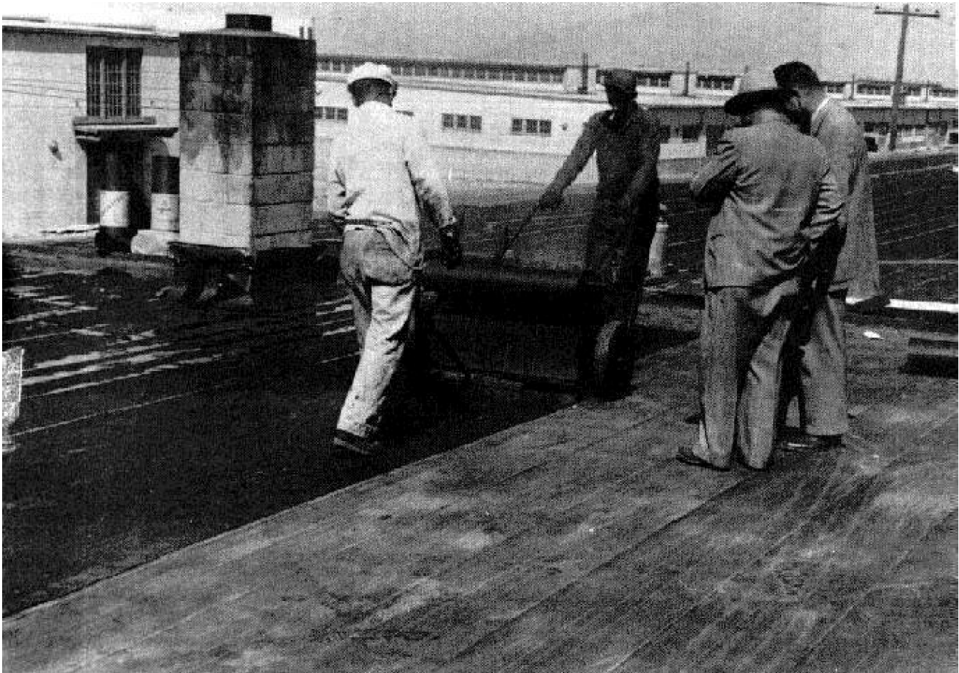
Figure 9. Laying felts mechanically and brooming-in after felt is rolled into hot bitumen.
