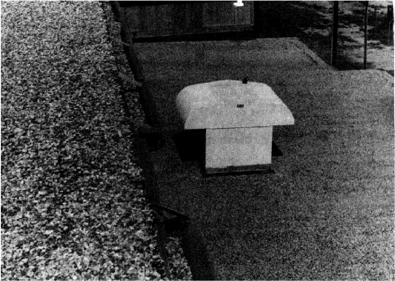
Figure 54. Accumulation of gravel causing collapse of gutter.
