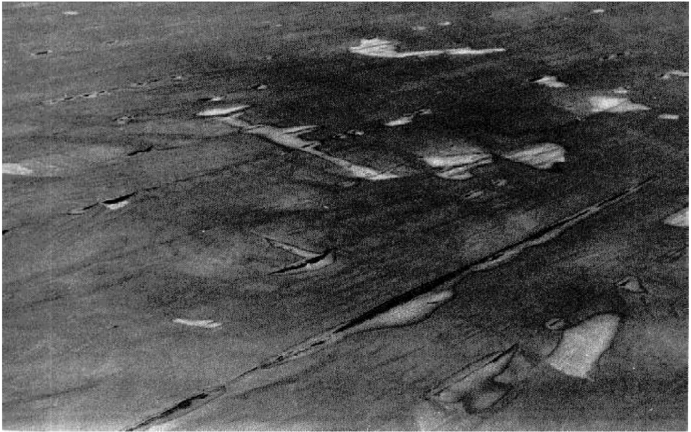
Figure 3. Wrinkles, buckles, lack of adhesion of felts.
