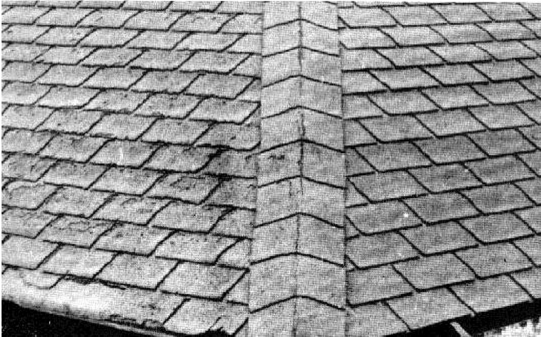
Figure 24. Difference in weathering of asphalt shingles on southern and eastern exposures.
