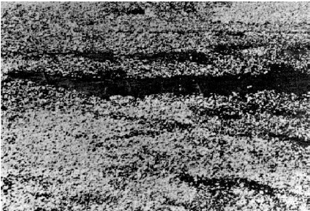
Figure 14. Felts exposed and weathered due to loss of aggregate and bituminous coating.
