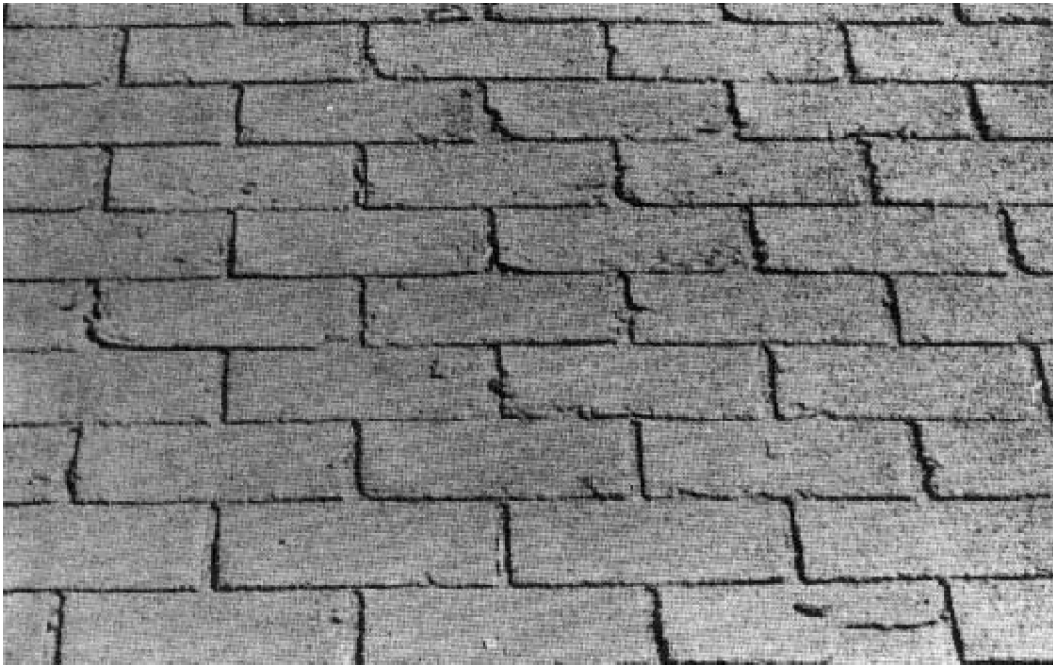
Figure 27. Recoated asphalt shingles — note damage resulting from brittleness.
