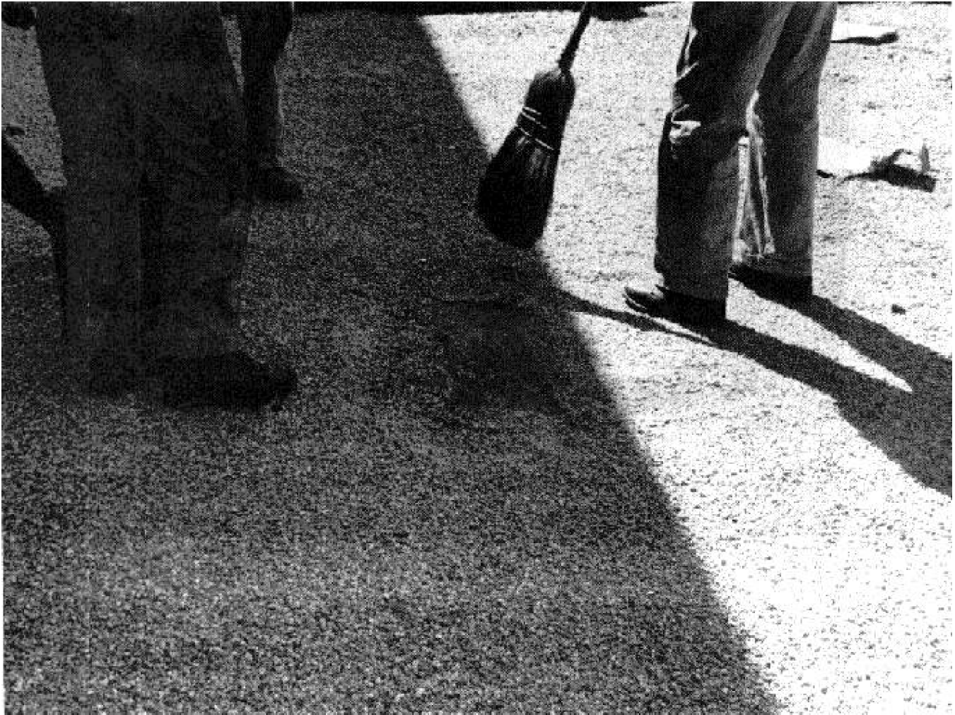
Figure 11. Insufficient bitumen to embed aggregate surfacing.
