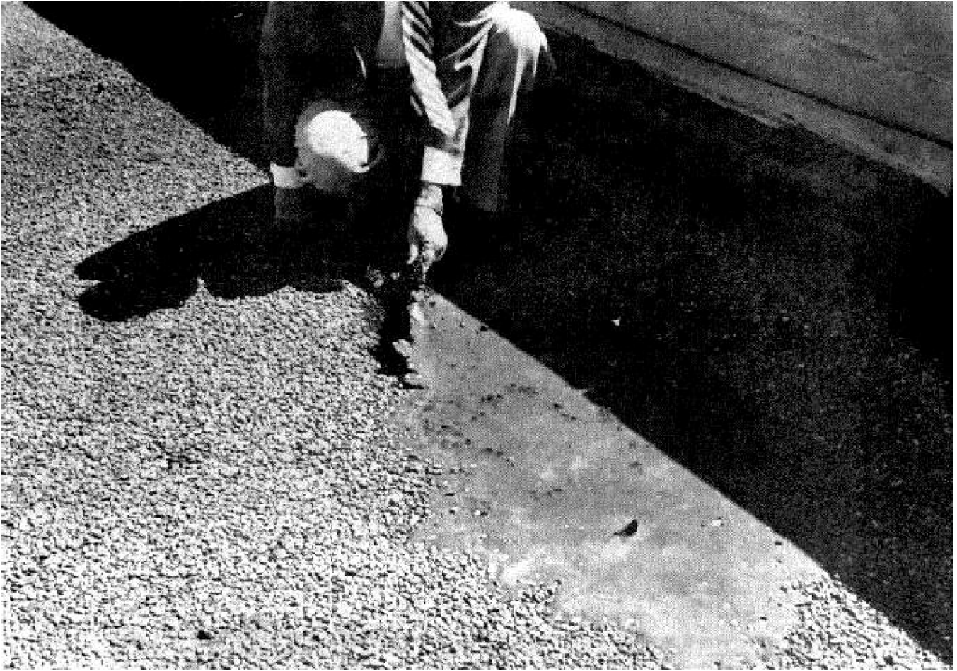
Figure 13. Hot bitumen poured on unprepared surface — note lack of adhesion.
