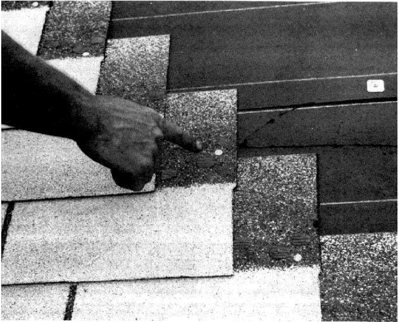
Figure 4. Asphalt shingles nailed too high.
