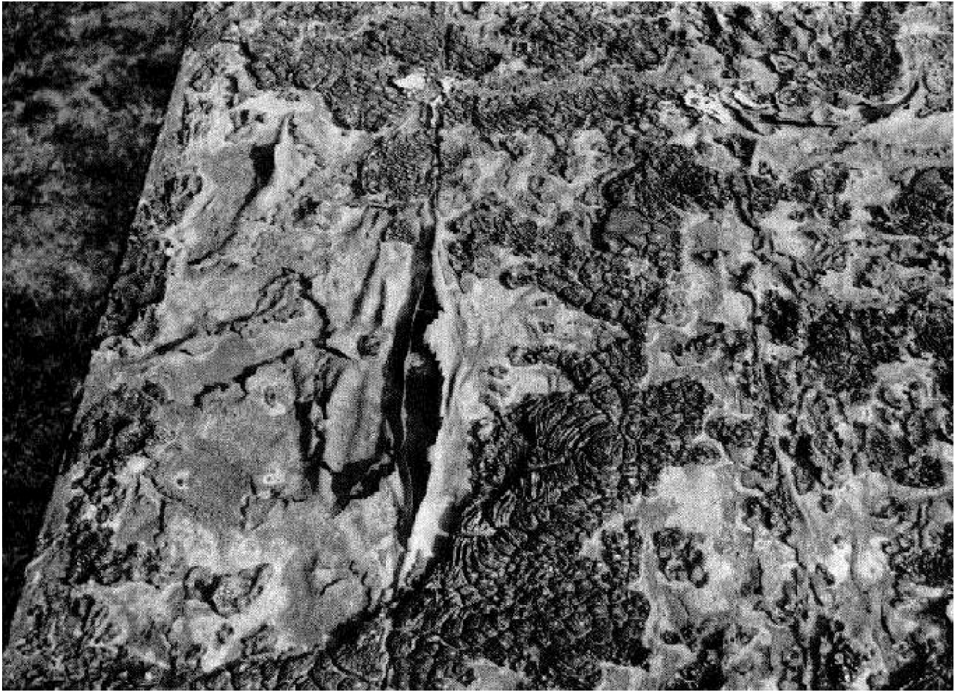
Figure 20. Felts disintegrated and disbonded — reroofing is mandatory.
