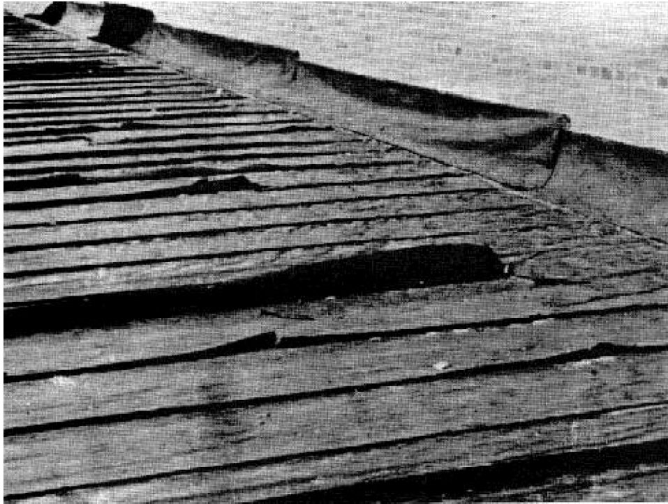
Figure 8. Results of poor workmanship in applying built-up roof.
