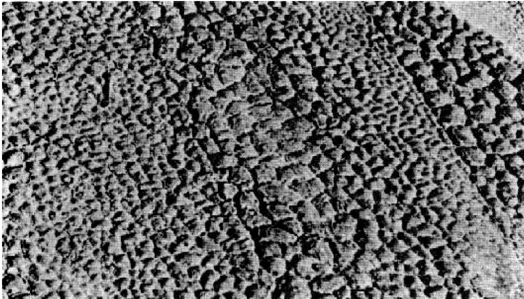
Figure 17. Alligatoring and cracking of a cold coating over alligatoring asphalt surface after 1 year exposure.
